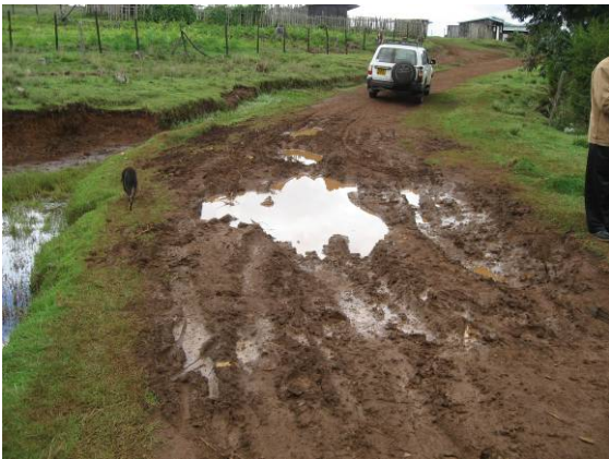
Figure 14. The road situation before the maintenance, in September 2008 (Kenya)
